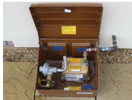
A typical meter box - open
