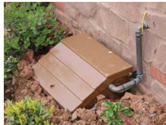
A typical meter box - closed
